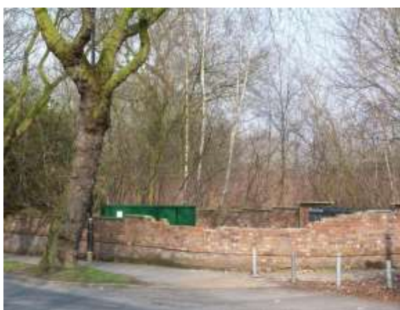
Substation and damaged wall on the east side of Redclyffe Road
